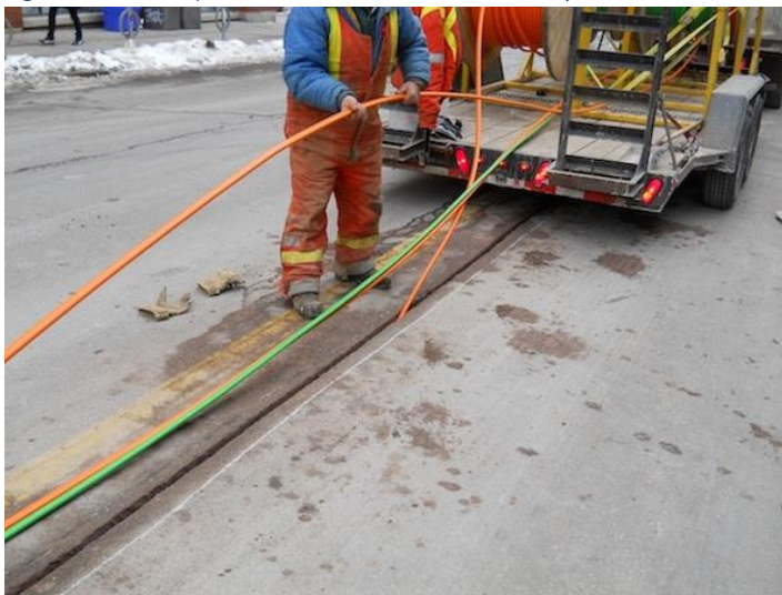
Figure 13 - Fibre Optic Cable Installation in a Roadway
