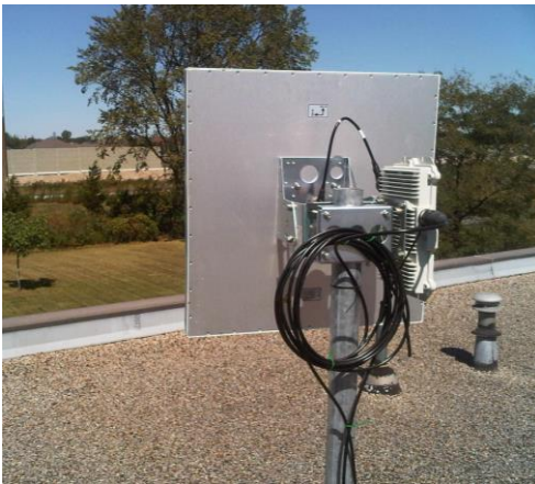
Figure 17 - Typical Fixed Wireless Antenna
