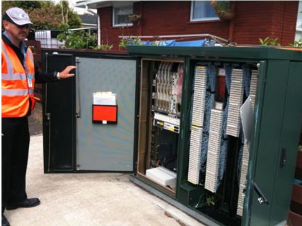
Figure 5 - DSL Cabinet in a neighbourhood
